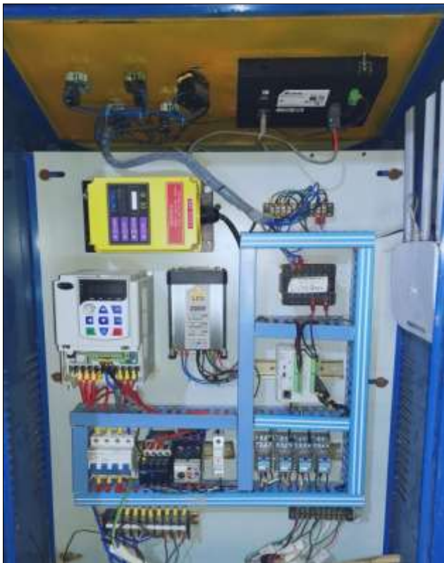
Fig 10: Main control board
